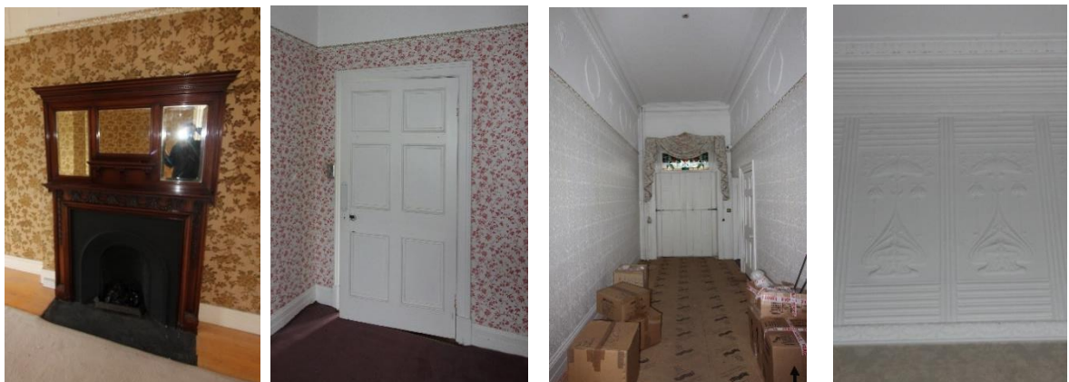
Fig.15.16: Late 19 th century fire piece (L), typical door joinery (M), cornice & frieze details (R)
